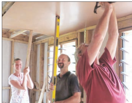
Zsofi and Miklos hold the ceiling sheet in place while 2nd Peter nails
